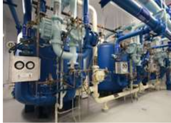
Ion Exchange – Romeoville, IL
