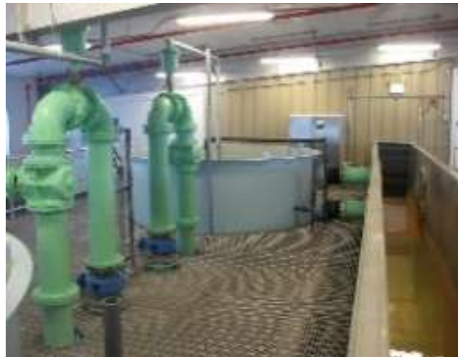
Fluidized Bed Reactors – Bargersville, IN
