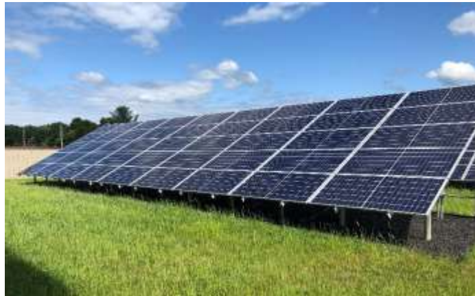
Ground Mounted PV Array
