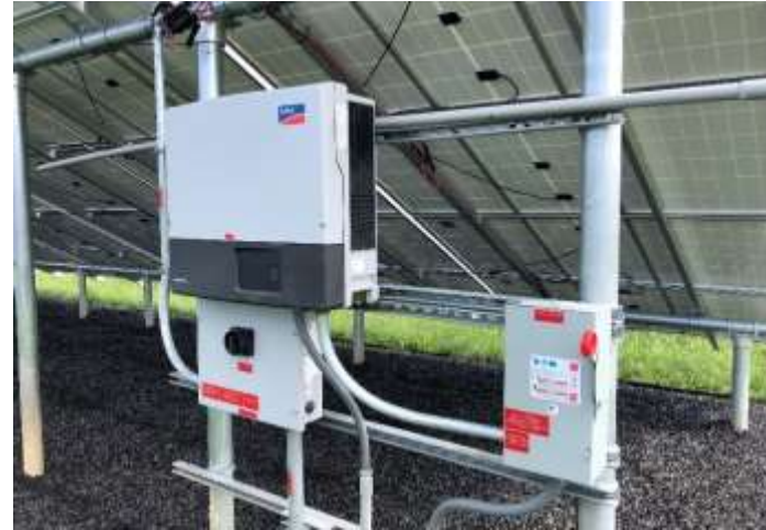
Solar Inverter and Disconnects
