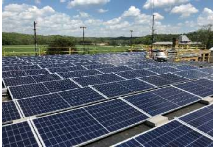
Roof Mounted PV Array
