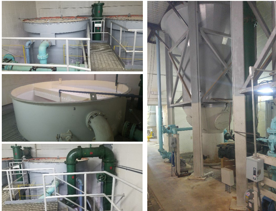
Existing Fluidized Bed Reactors at HECLA Water Treatment Plant. Renovations to fluidized bed reactors and conversion of facility from lime to caustic soda for pH control are currently under design by Strand.
