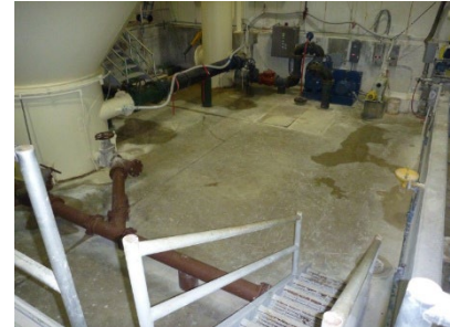
The small footprint and modular installation of the ion exchange units will be placed in CU's existing treatment building with no building expansion required.
