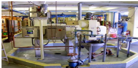
Installed lime slaker with automated gravimetric feed.
