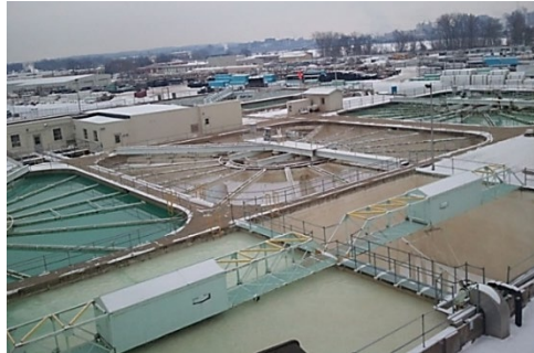
Lime softener clarifier basins.
