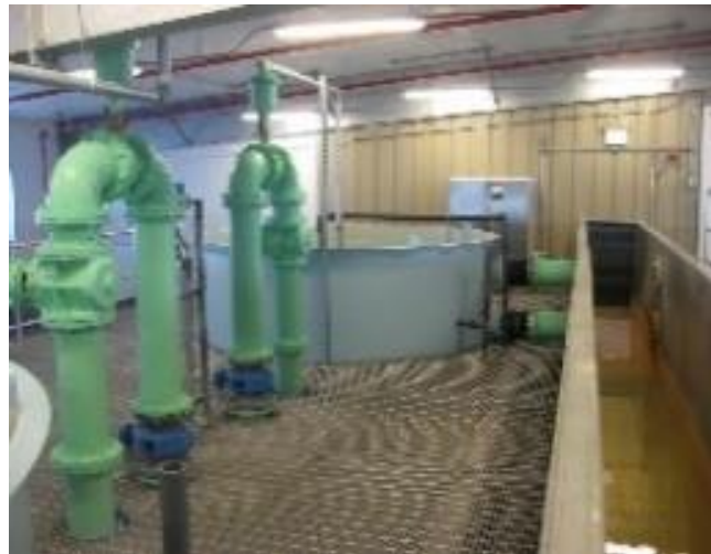
Fluidized Bed Reactors – Bargersville, IN
