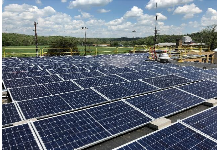
Roof Mounted PV Array
