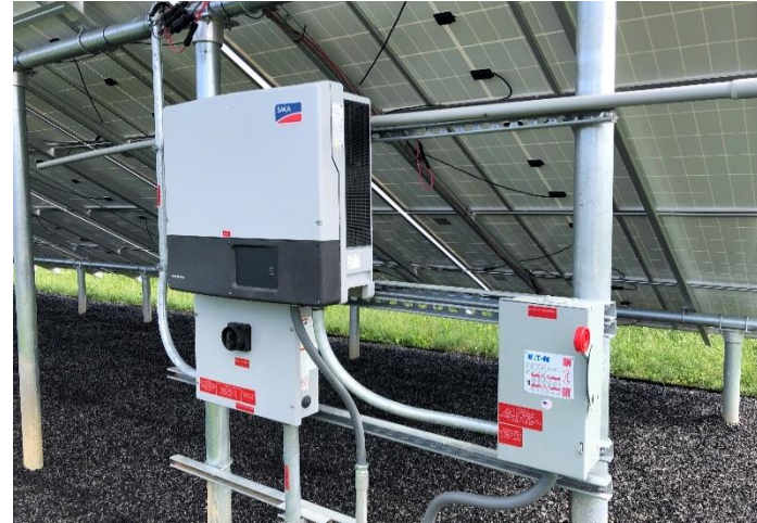
Solar Inverter and Disconnects
