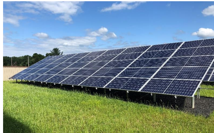
Ground Mounted PV Array
