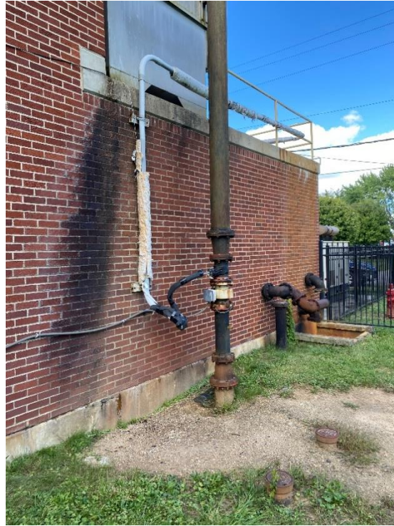
Figure 2: Chlorine Feed Point
