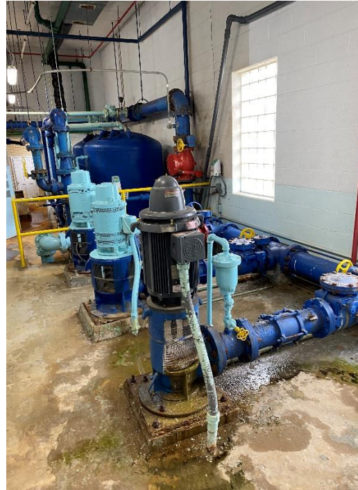
Figure 8: High Service Pumps
