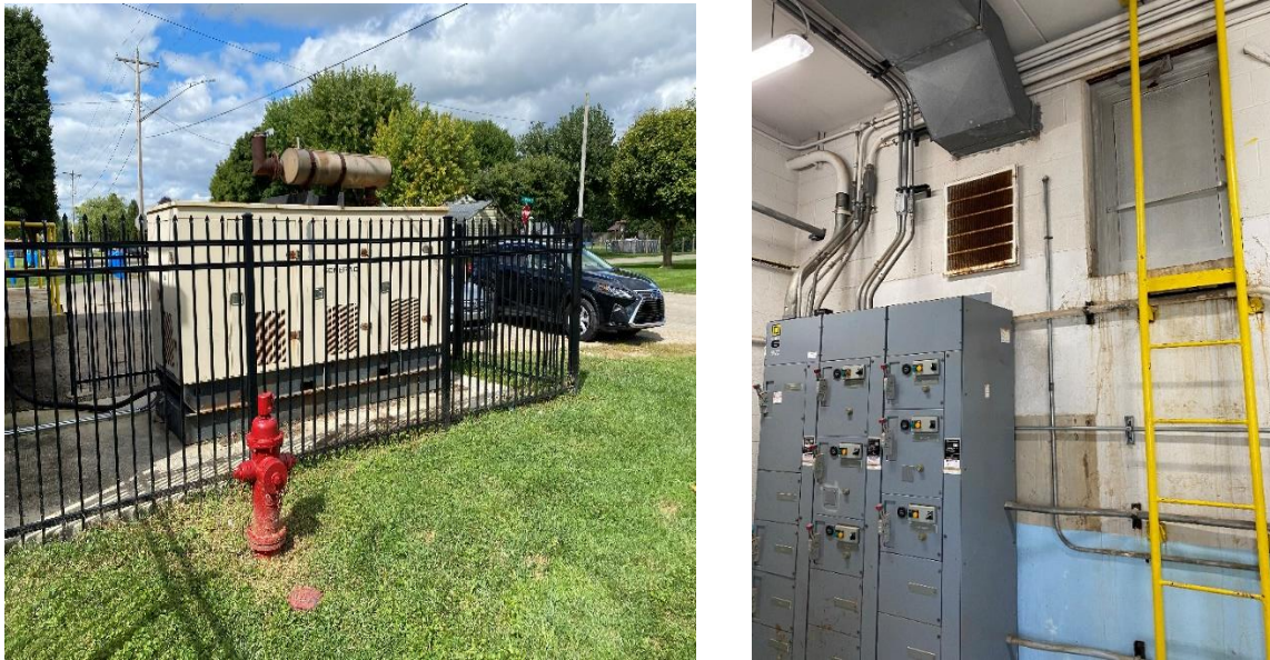
Figure 11: Generator and Electrical Control Panel
