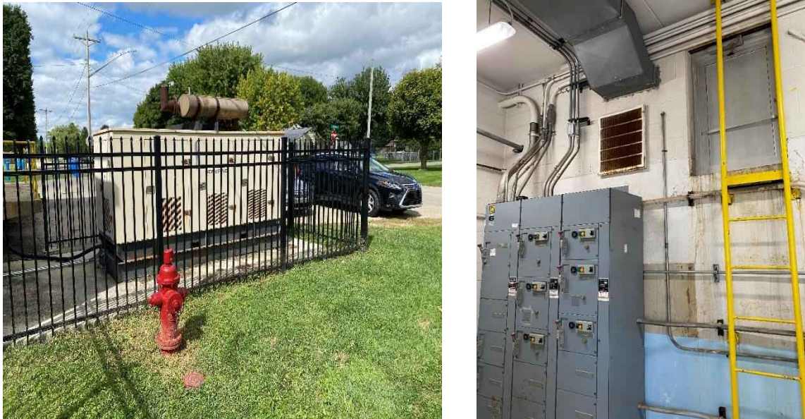
Figure 11: Generator and Electrical Control Panel
