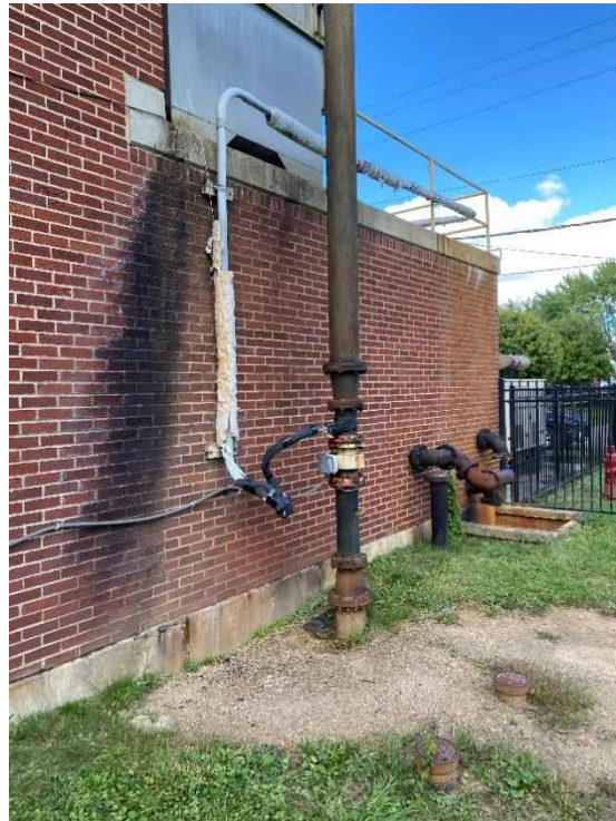
Figure 2: Chlorine Feed Point
