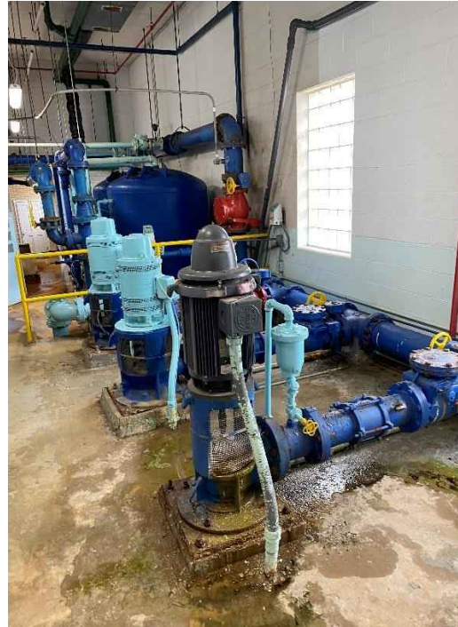
Figure 8: High Service Pumps
