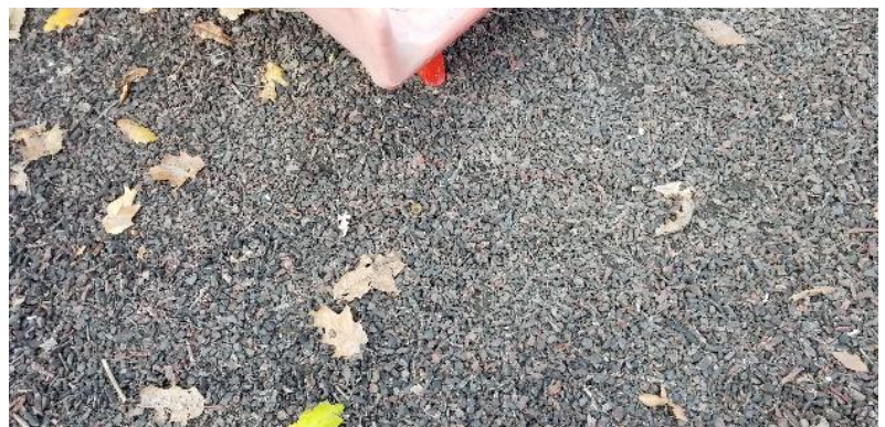
Surfacing is too thin (lacking proper depth). Concrete footers are exposed.
