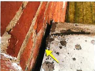
Existing coping is thin gauge aluminum, and not properly installed. It has gaps in seams that allow water and snow to blow underneath. New commercial 26 gauge coping needs installed on parapet wall.
