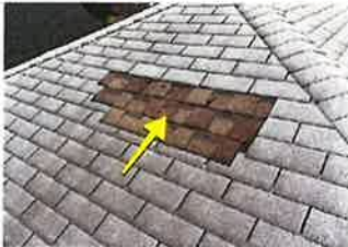
Incorrect patch job. Wrong kind of shingles, wrong size of shingles, wrong color of shingles
