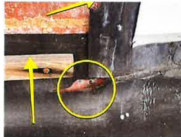
Not properly fastened to brick wall, this catches the water and causes it to drain into the building. Rubber needs lapped up the brick wall and term bar installed with proper commercial sealant.
