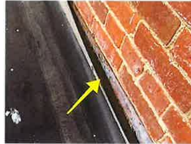
Not properly fastened to brick wall, this catches the water and causes it to drain into the building. Rubber needs lapped up the brick wall and term bar installed with proper commercial sealant.
