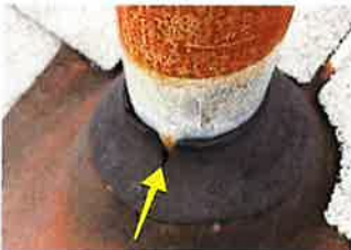
Flashed rings around pipe boots are deteriorated and cracking
