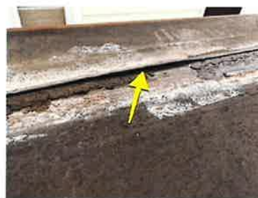
Due to the age of the EPDM, the seams are completely delaminating and deteriorating. This allows water to run right between the seams and reach the roofing deck, causing deterioration and water damage on the inside of the building.
