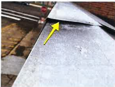
Existing coping is thin gauge aluminum, and not properly installed. It has gaps in seams that allow water and snow to blow underneath. New commercial 26 gauge coping needs installed on parapet wall.
