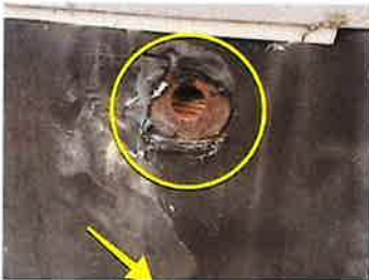
Exposed hole through the rubber on the parapet wall.
