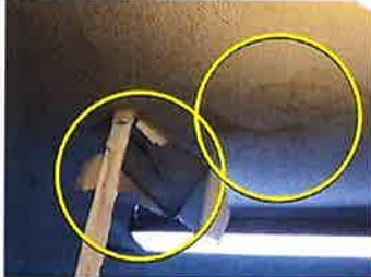
Interior water damage due to the rubber roof leaking. This rubber roof has surpassed its life expectancy and is deteriorating and leaking in many areas.
