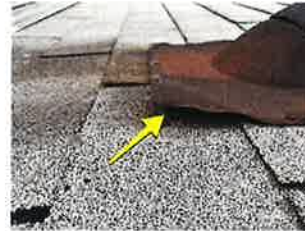
Problems are fixed, which allows water and wind to blow underneath and cause a leak.
