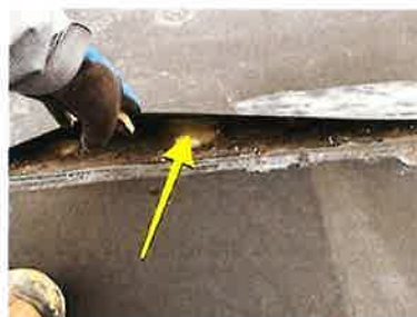
Due to the age of the EPDM, the seams are completely delaminating and deteriorating. This allows water to run right between the seams and reach the roofing deck, causing deterioration and water damage on the inside of the building.
